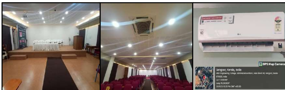
HVAC facilities observed in the Campus
